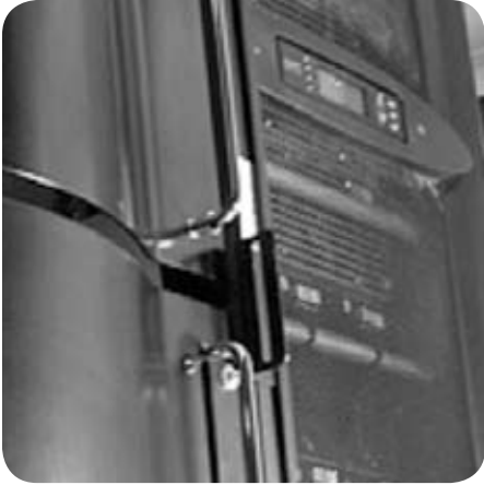
Photo courtesy of Hydrogenics Corporation
