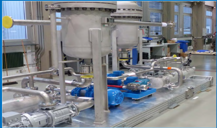
Final assembly of the Siemens electrolyser for Project Mainz, a joint energy storage project of Stadtwerke Mainz, Siemens, Linde, and RheinMain University. The system, equipped with an electrolyser from Siemens, will convert surplus electricity from wind farms to hydrogen. (Source: Siemens)
