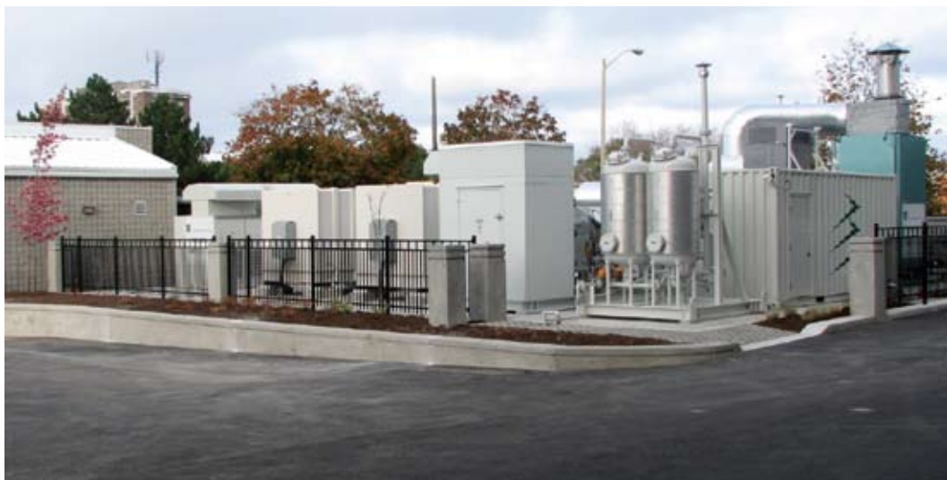
Photo: Enbridge Gas Distribution and Fuel Cell Energy | Direct Fuel Cell-Energy Recover Generation Power Plant in Toronto, Ontario
