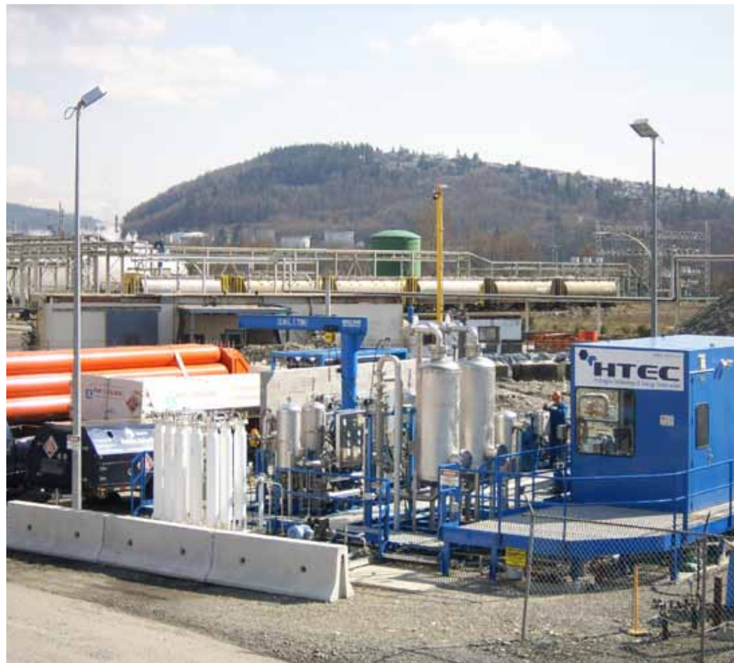
HTEC waste hydrogen capture facility in North Vancouver, BC
