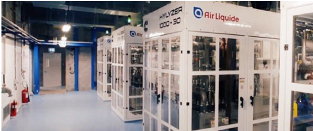
Figure 5: Electrolyzer modules at Air Liquide's 20MW green-hydrogen facility in Bécancour, Canada, support battery materials and existing industrial cluster in Quebec. Source: Air Liquide.
